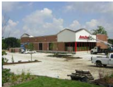
Pictured above: AutoZone, located at the northwest corner of Algonquin and Crystal Lake Roads opened August 24, 2007.
